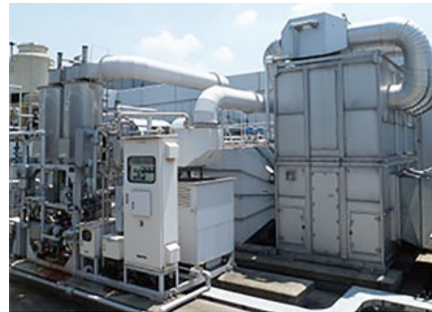
Organic solvent recovery equipment at Nara Research and Development Center
