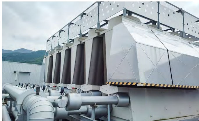
Air cooled chiller at the Shiga Product Supply Center
