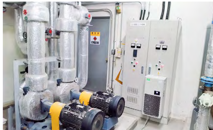
Chilled water backup circulation pump at the Shiga Product Supply Center
